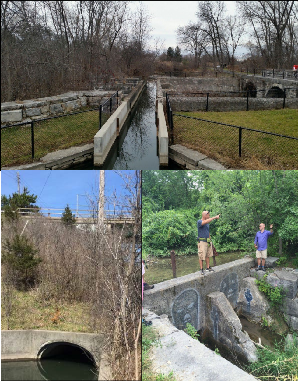
Photo 12. At top: The intact portions of the Butternut Creek aqueduct (facing east) include the intact stone support structures and the recently repaired spillway; the location of the missing wooden sluice would be between the spillway and the Canalway Trail on the far right of the image. Bottom left: Water levels and circulation are supported (or hindered) by the connection to the Orville Feeder Canal through culverts under I-481; additional hydrological analysis is required to understand the capacity of the infrastructure to sustain additional water flow. Bottom right: Restoration of the sluice gate on the Orville Feeder Canal is a recommended canal infrastructure improvement, though this initiative also requires additional hydrological analysis for its potential impacts on Butternut Creek.
