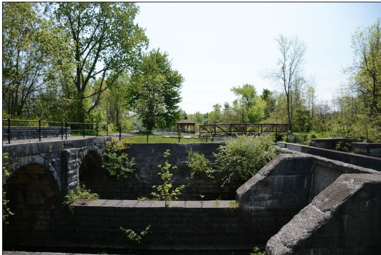
Photo 1: Aqueduct near the existing terminus of the Erie Canalway Trail, view looking east toward Cedar Bay
